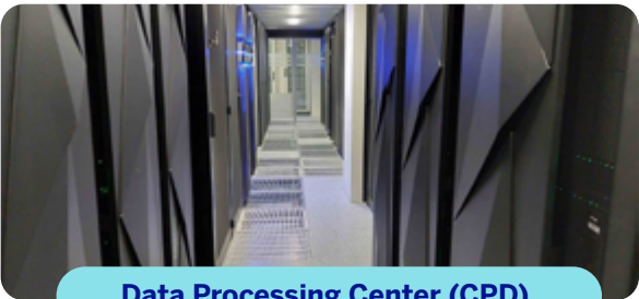
Data Processing Center (CPD)
