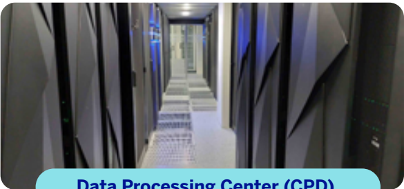
Data Processing Center (CPD)
